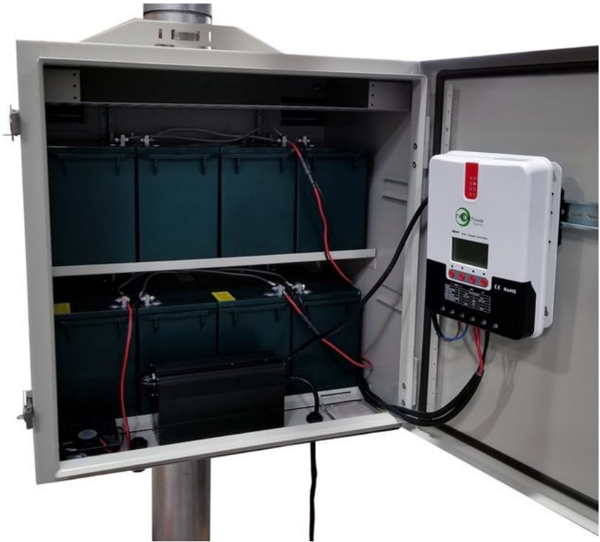
UPS-STL-600 8 Battery System
