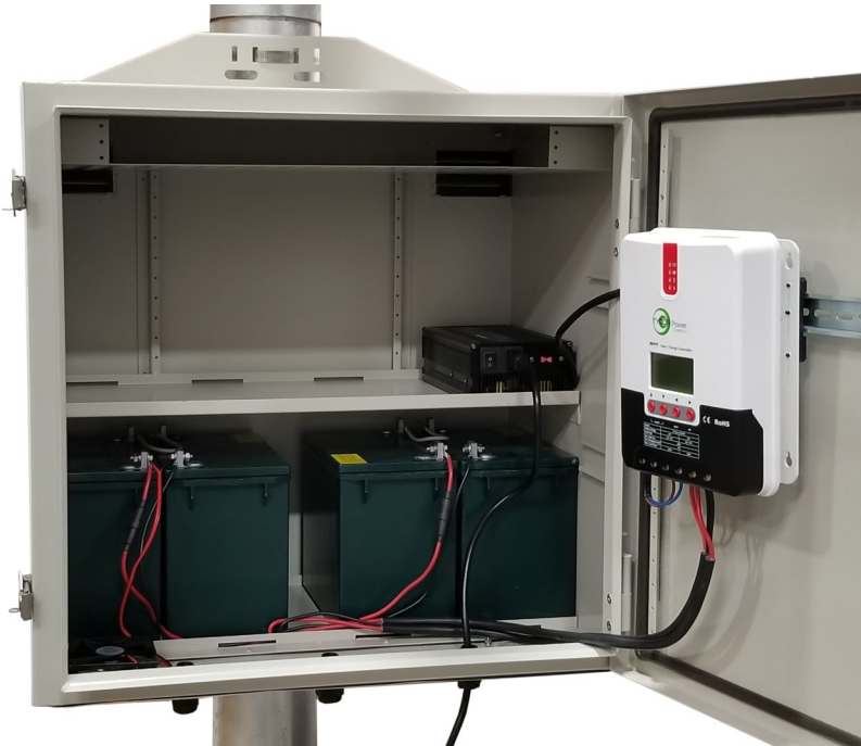
UPS-STL-600 4 Battery System
