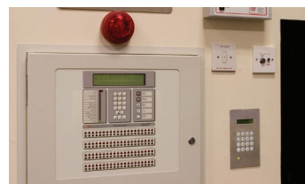
Fire Alarm Systems
