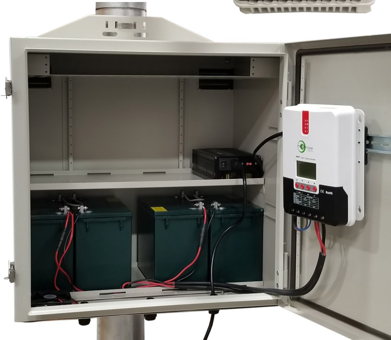
UPS-STL48-600 4 Battery System
