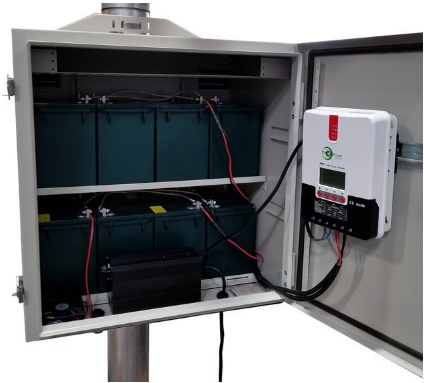
UPS-STL48-600 8 Battery System
